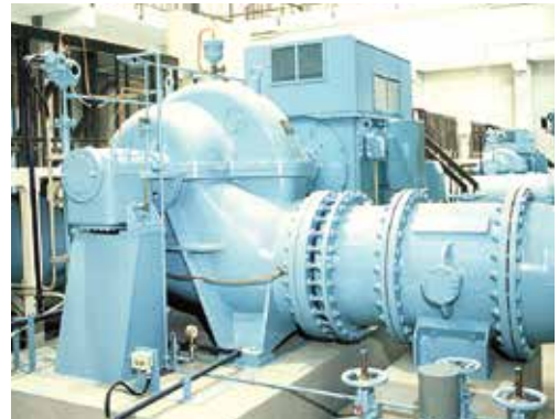
Irrigation Pump CDM800×600mm, 4,200m 3 /h, 60m, 900kW
