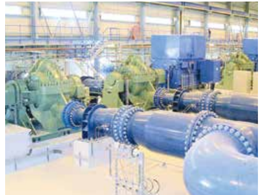
Potable Water Transmission pump CDM800×500mm, 4,740m 3 /h, 250m, 4,700kW
