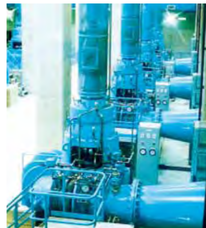
Intake pumps in city water plant (size : 800mm), Hong Kong
