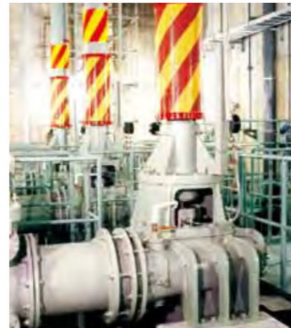
Sewage pumps (size : 450mm), Japan
