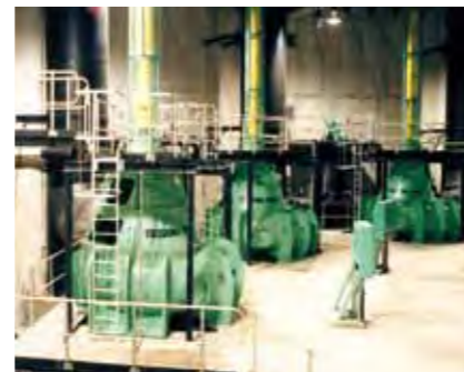
Sewage pumps (size : 1,300 × 1,100mm), Hong Kong
