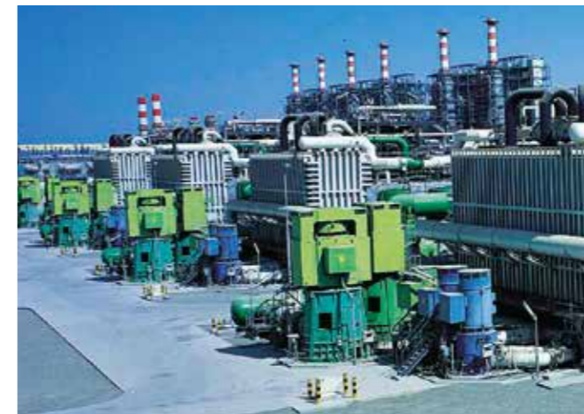
Various seawater pumps in Al Taweela MSF desalination plant, Abu Dhabi, UAE
