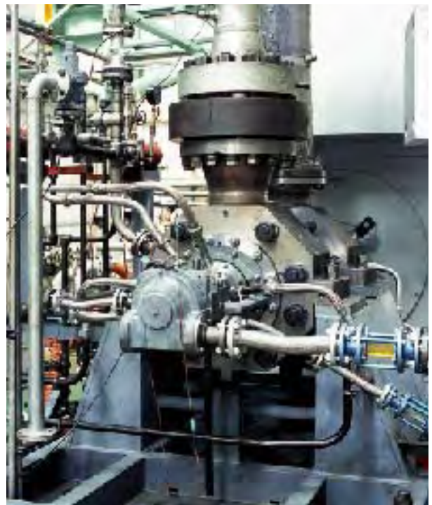
Segmental ring-section casing boiler feed pump 3,018ft-2,100 U.S.gpm-2,980min -1 -2,050HP Fujairah Power Plant(Abu Dhabi), 660MW
