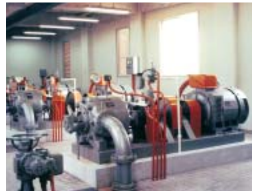
Distributing pumps in small-capacity water works
